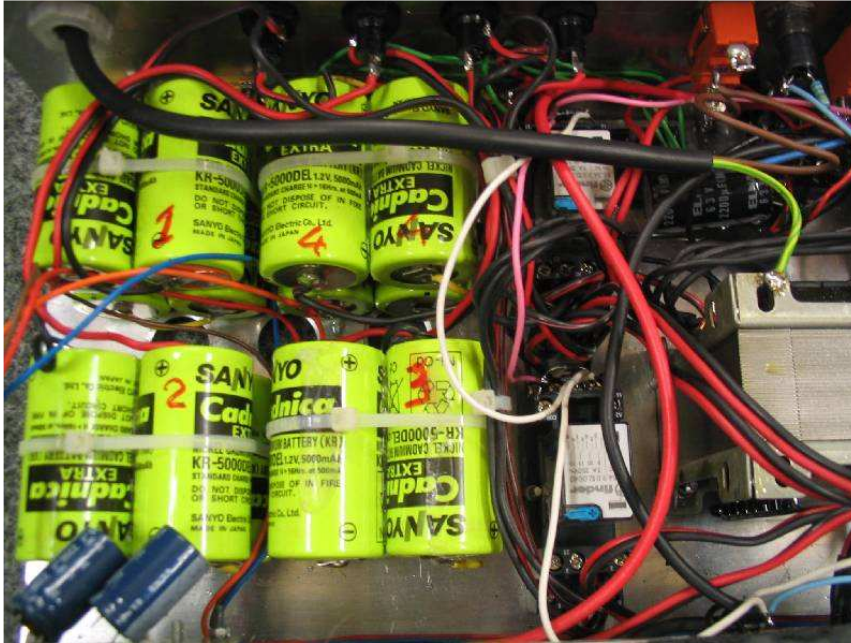
Figure B-11: Particular of the power supply box: battery groups 1 to 4 are shown together with tension regulators and 2 relays.
