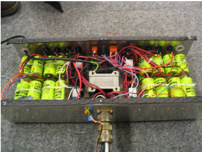
Figure B-10: Inside of the power supply box: from the 8 groups of 4 batteries the power supply passes through the red and violet cables, placed on purpose in those positions. The transformer which provides power supply for the digital part (in acquisition state) and recharges the batteries (in recharging state) appear in the center of the box.
